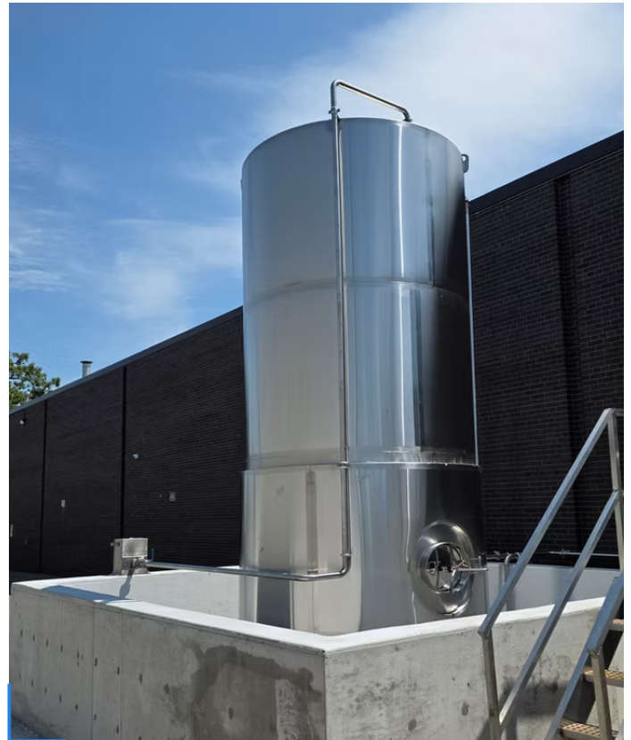
Heated, insulated outdoor storage silo.
